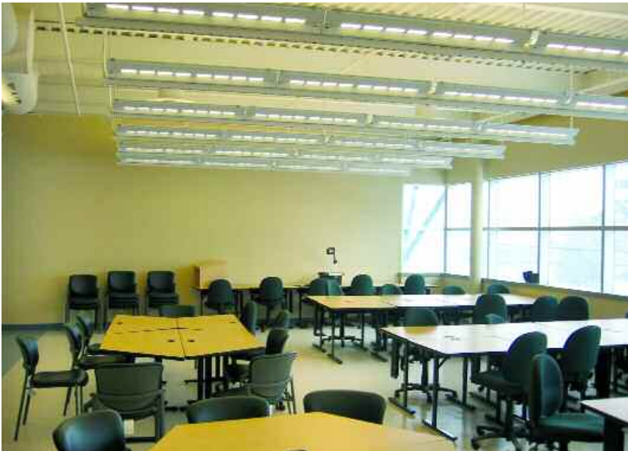
Exposed steel deck and beams at Nova Scotia Community College Pictou Campus. Design by Fowler Bauld & Mitchell Architects.
