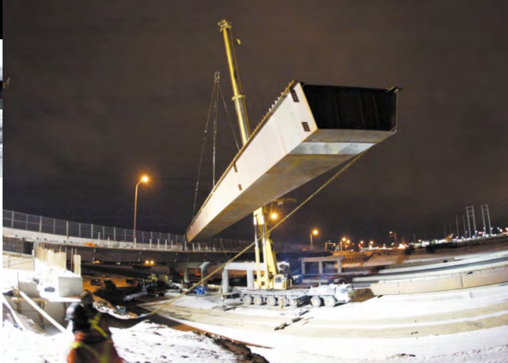
Present Owner: Region of Peel and Ministry of Transportation Ontario Structural Engineer: Giffels Associates Ltd. General Contractor: Fermar Paving Structures Subcontractor: Soncin Construction Steel Fabricator: Central Welding & Iron Works
